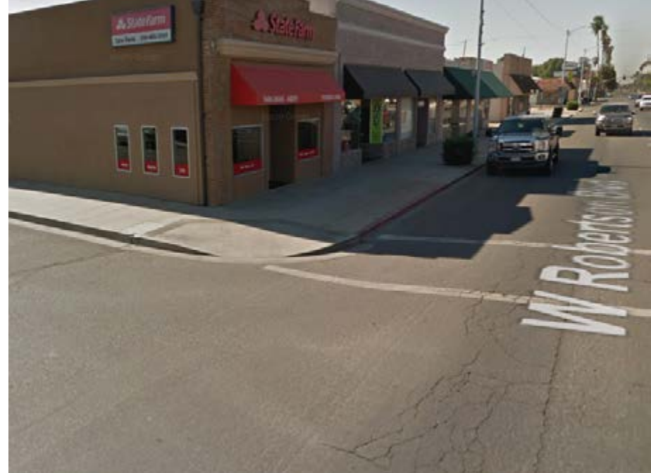
Curb ramp does not align with crosswalk at intersection of Robertson Boulevard/3rd Street. Source: Google Maps
