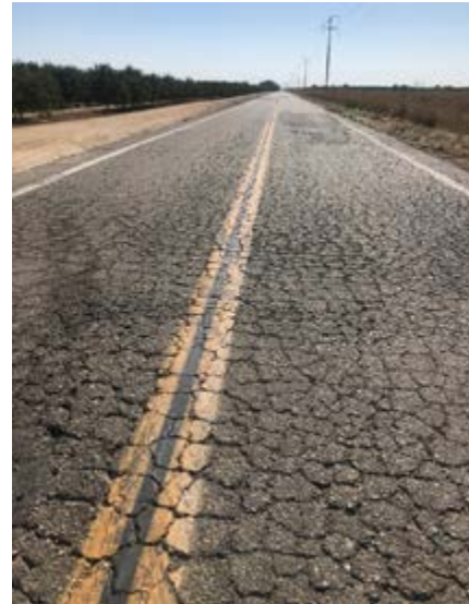
Alligator Cracking on Avenue 26 near Road 19
