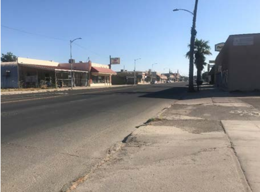
Sidewalk is not maintained near intersection of Robertson Boulevard/5th Street. Source: TJKM
