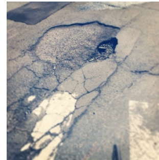
Poor pavement quality in a bicycle lane
