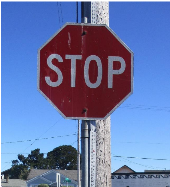
A sign which passed the retroreflectivity test but is damaged.
