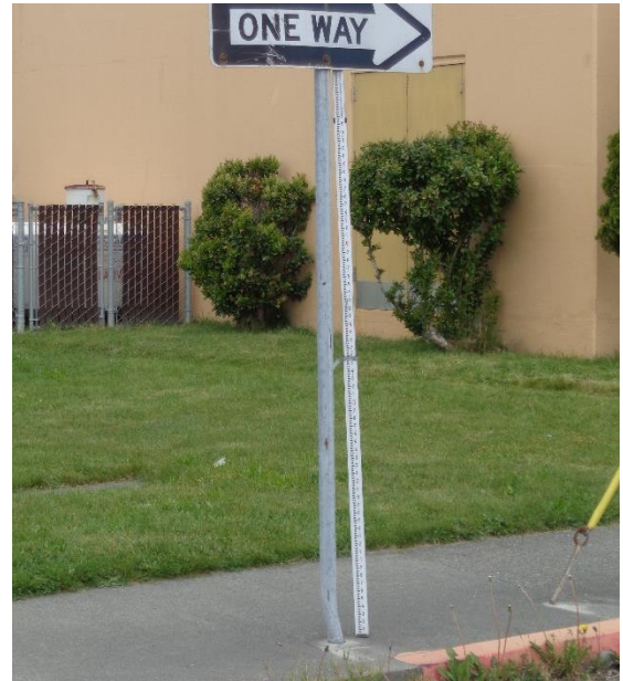
A sign post which is damaged and needs replacement.
