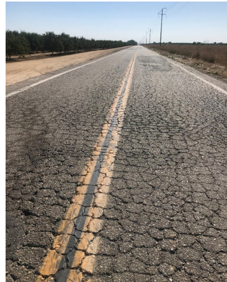
Alligator Cracking on Avenue 26 near Road 19
