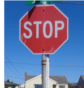
A sign which failed the retroreflectivity test.AA
