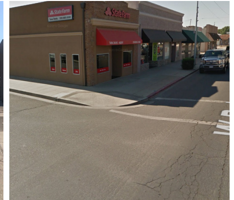
Curb ramp does not align with crosswalk at intersection of Robertson Boulevard/3rd Street.
