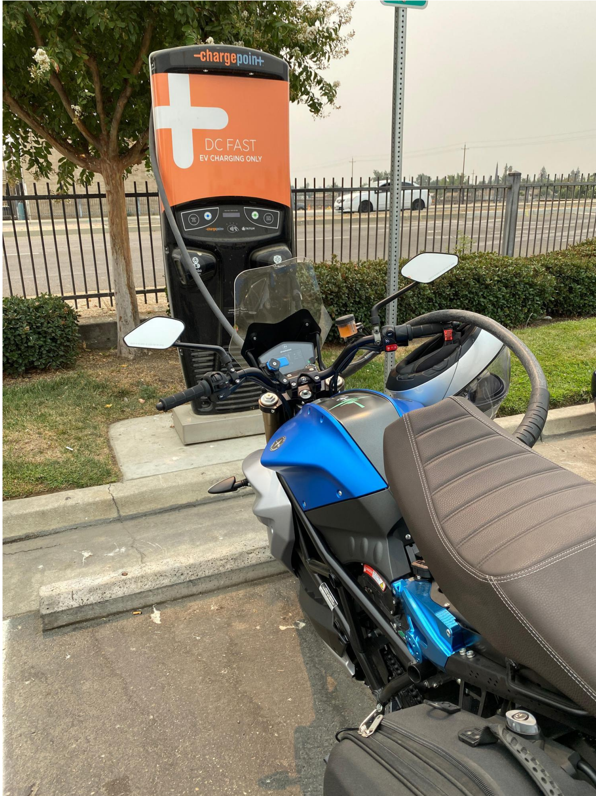
FIGURE A-9: CHARGEPOINT DC CORRIDOR SITE WITH A DC FAST CHARGER & L2 CHARGER (DUAL PORT), 105 CHOWCHILLA BVD, CHOWCHILLA (PHOTO: PLUGSHARE)
