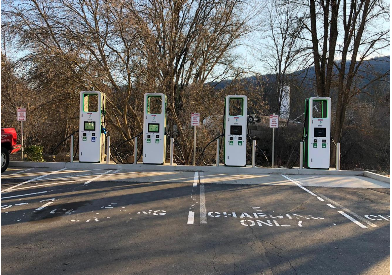
FIGURE A-7: 4 EVGO DC FAST CHARGERS, OAKHURST (PHOTO: PLUGSHARE)
