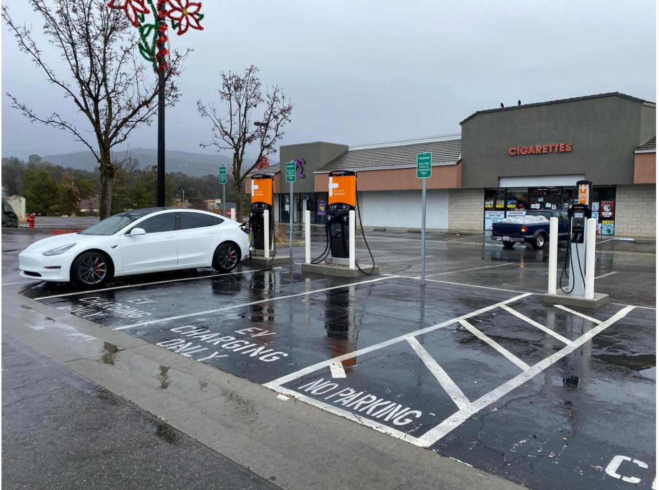
FIGURE A-6: 2 DC FAST AND 2 LEVEL 2 CHARGERS, NEAR JACK IN THE BOX, 40050 CA-49, OAKHURST (PHOTO: PLUGSHARE)
