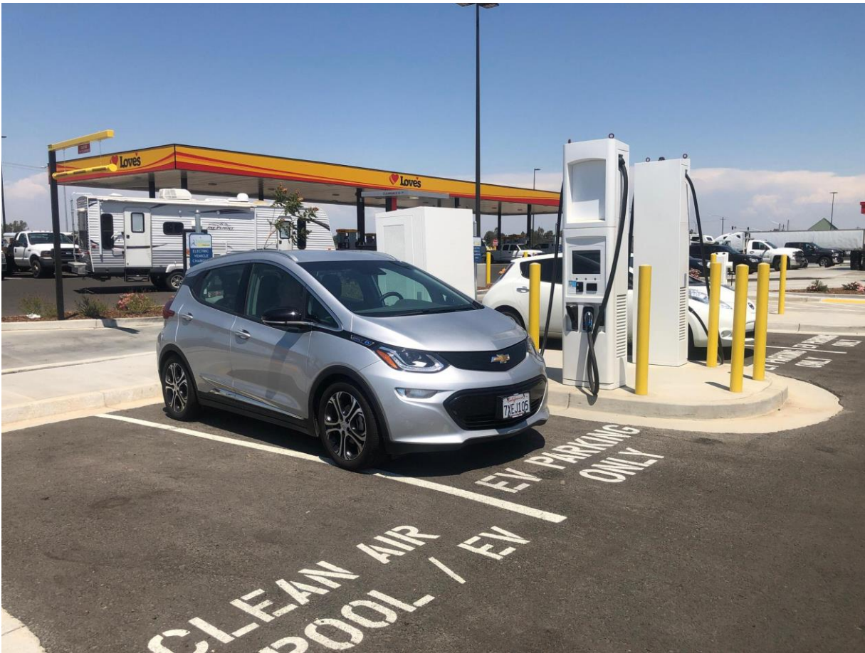
FIGURE A-11: 2 EV CONNECT DC FAST CHARGERS, 1750 AVENUE 17, MADERA (PHOTO: PLUGSHARE)
